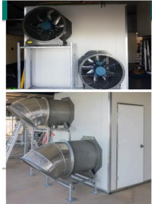
Figure 10: One of DC2's active regional modular data centre
